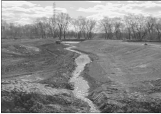
An unnamed 800-foot stream on the project site flows into Raritan River. Banks have been contoured to prepare for planting of Willow trees. Credit: Mike Breslin, Contractor, Green Brook Project.
