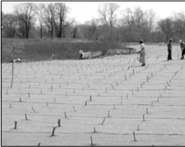
Thousands of "Willow Stakes" are planted in burlap weed barriers along side the stream. Credit: Mike Breslin, Contractor, Green Brook Project.
