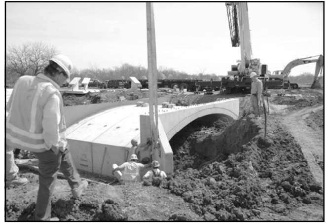
Multi-section pre-cast concrete bridge is lowered by crane across stream. Bridge leads to visitor parking area where nature walkway begins. Credit: Mike Breslin, Contractor, Green Brook Project.
